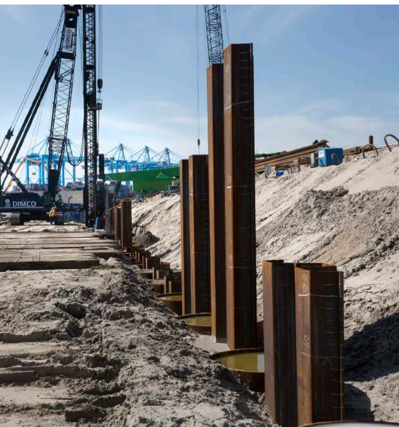
Rotterdam - The Netherlands Works were successfully concluded at the Offshore Terminal Rotterdam
