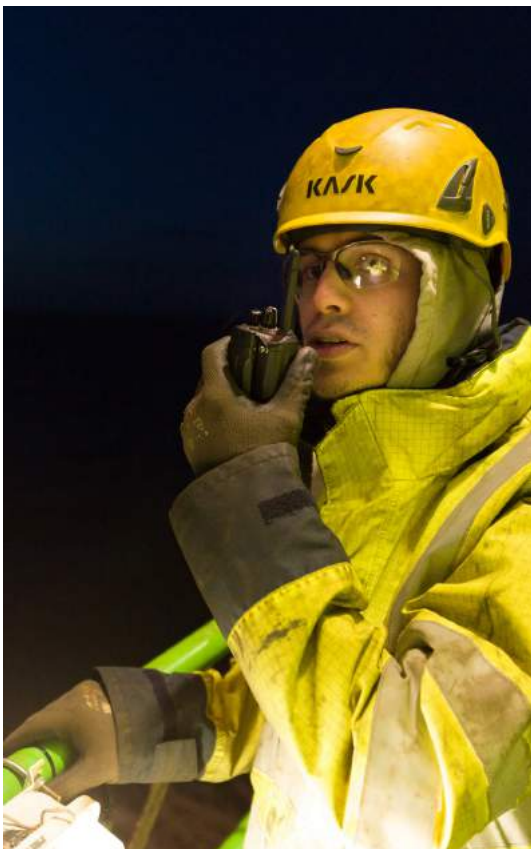
UK 56 foundations were installed well ahead of schedule at the Galloper offshore wind farm
