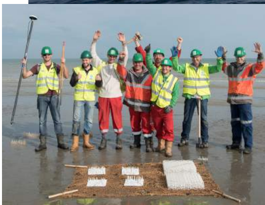
De Panne - Belgium Coastbusters installation of eco-friendly reefs to prevent coastal erosion
